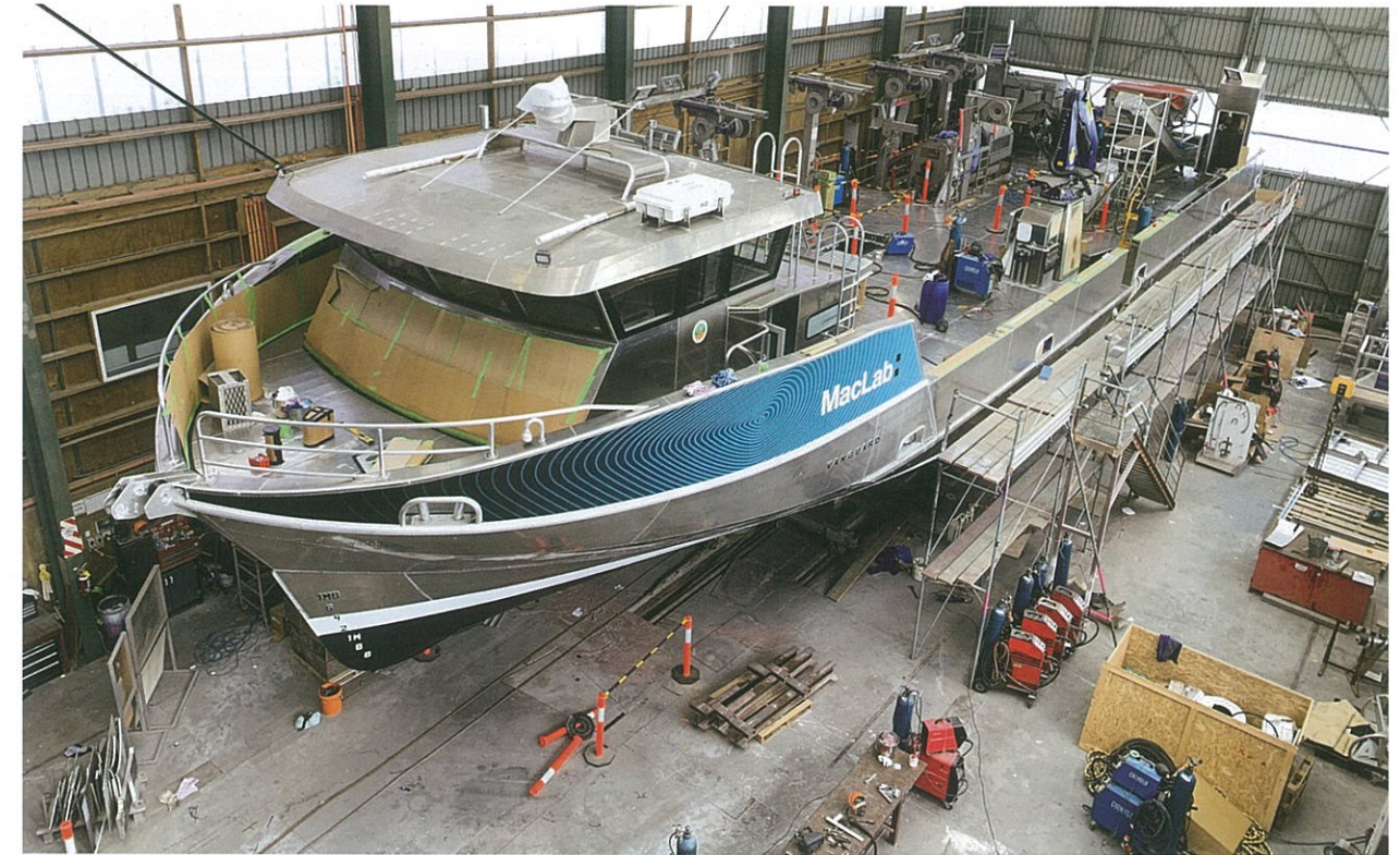
Vanguard’s hull was built upside down, then flipped using four cranes before construction continued inside the shed.
